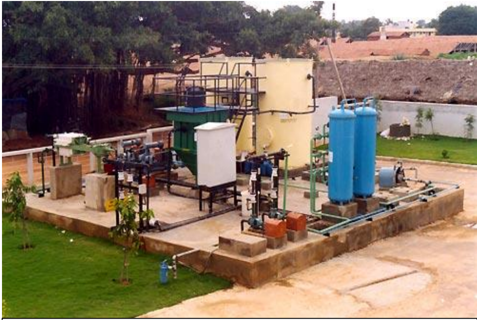
Effluent Treatment Plant
