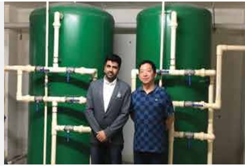
WTP at "MANSION DE SALAM" A Leed Gold Certified Green Residential Project
