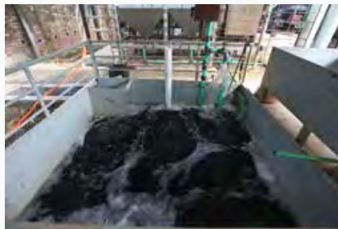
KARAMTOLA GENERAL HOSPITAL ETP & STP (capacity 50 m 3 /day)
